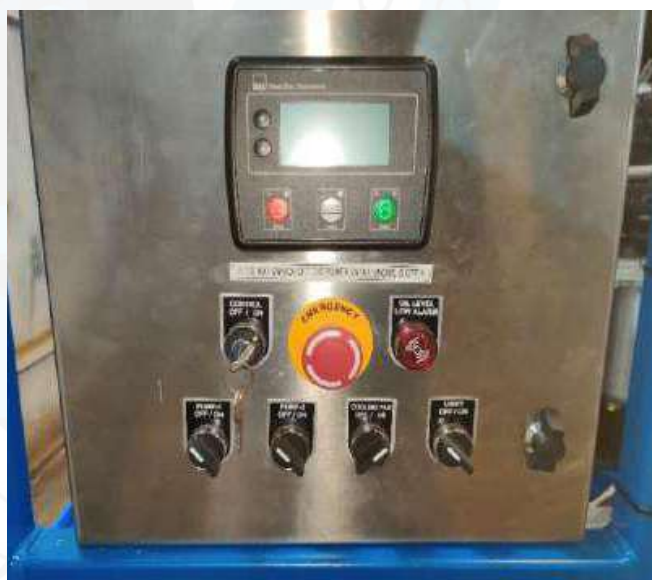
ENGINE CONTROL PANEL
